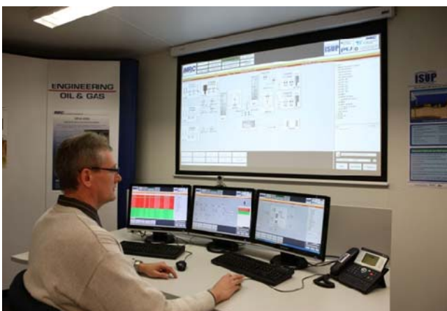
Figure 2: Local Control Room with web based SCADA (IMPac)
